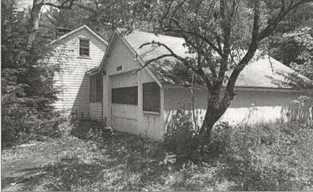
Photo 1: View of garage attached to house
