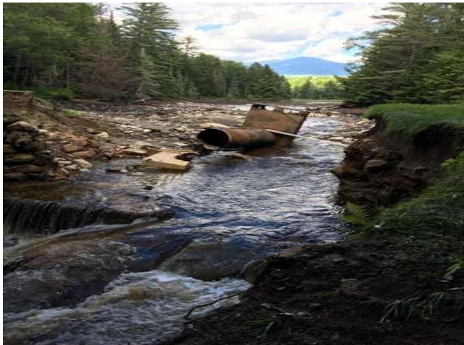
Photo 2: Looking northeast at failed Weeks dam and washed-out Gould Hill Road in 7/2017.
