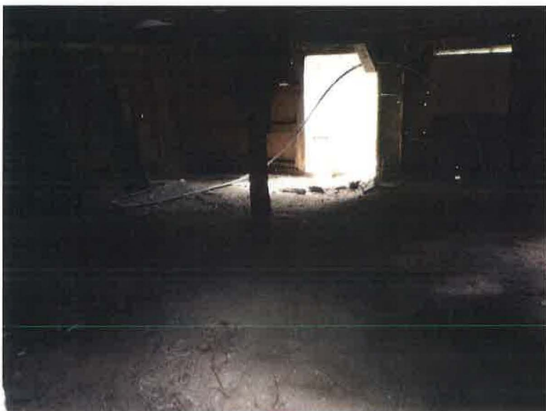
Building looks like a two story building but no way to get to the second floor. Old concrete floor.
